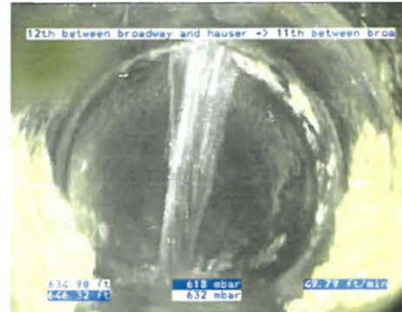
▲ Infiltration Gushing Through Pipe Joint
