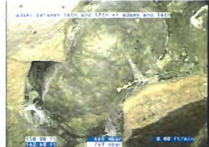
▲ Large Hole in Sewer Pipe with Large Rock Above Hole
