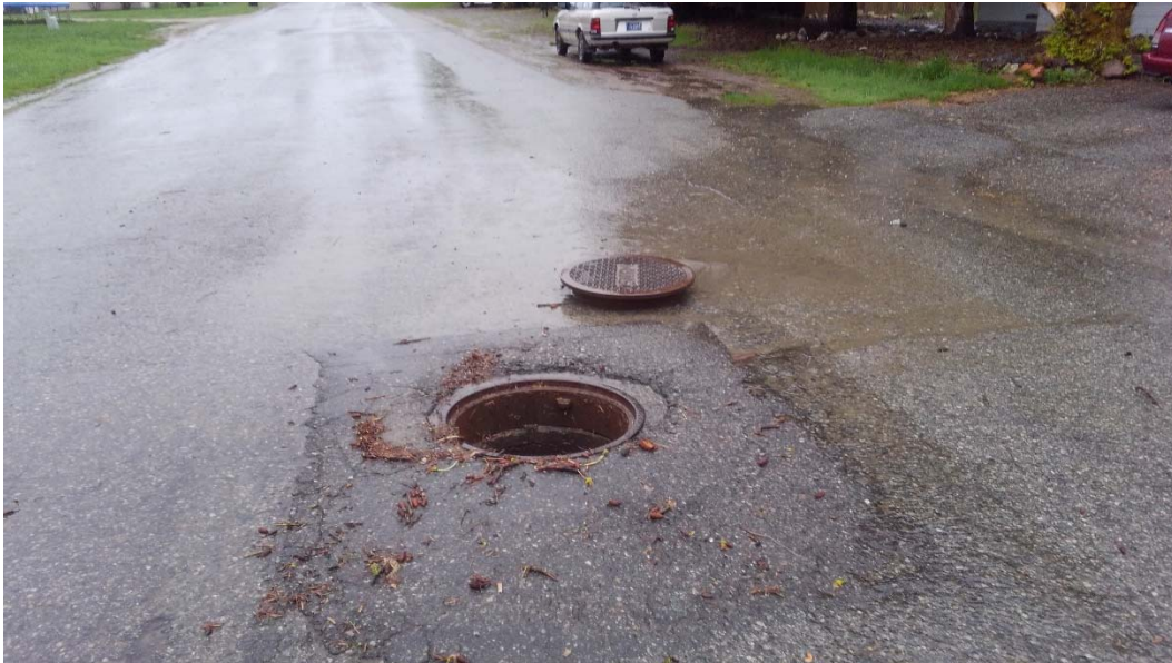
Manhole cover blown off during May 22 rain event, 3 rd and Haggin.
