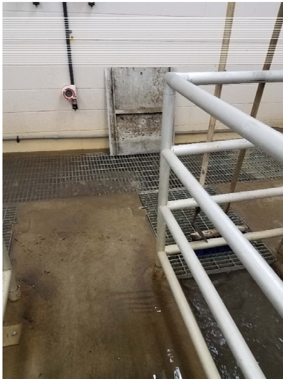
Inflow to sanitary sewer treatment plant during rain event. Contaminated water flooding building and bubbling out of grates.
