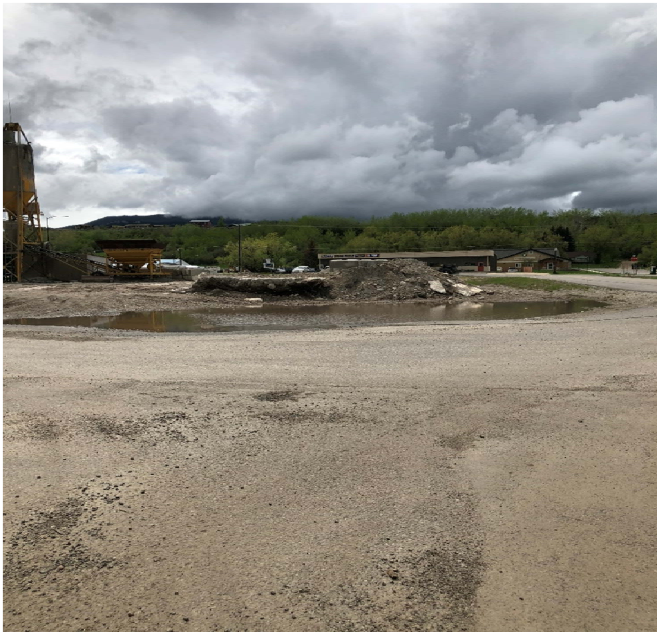
Localized flooding at north end of Haggin Avenue, near MDT outfall.
