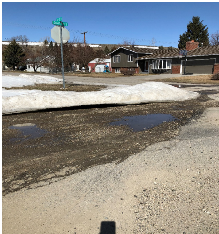
Resident identified flooding area at corner of 18 th Street and Grant Avenue.
