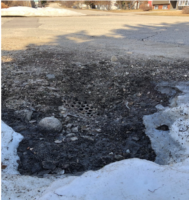
Typical storm inlet on existing infrastructure, cover has structural damage and is almost completely clogged.
