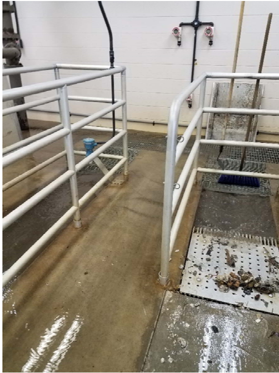
Inflow to sanitary sewer treatment plant during rain event. Contaminated water flooding building and bubbling out of grates.
