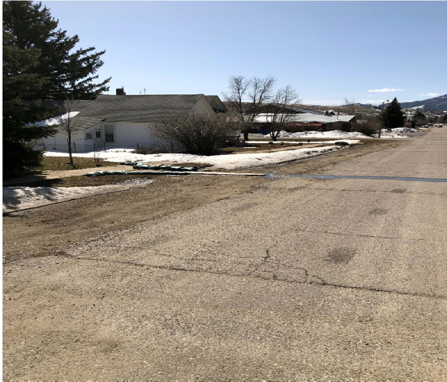
Drainage issues on Adams Avenue between 12 th and 13 th Street.
