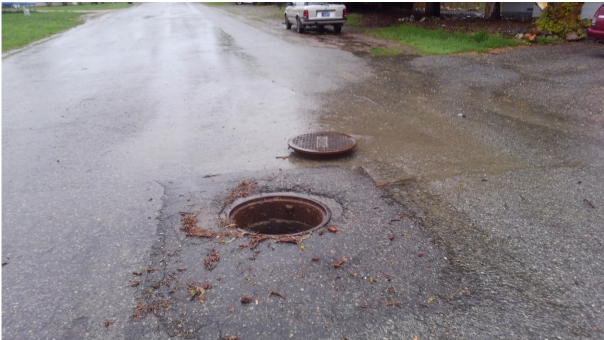
Figure 6: Manhole cover blown off by surcharging stormwater during May 22, 2018 storm
