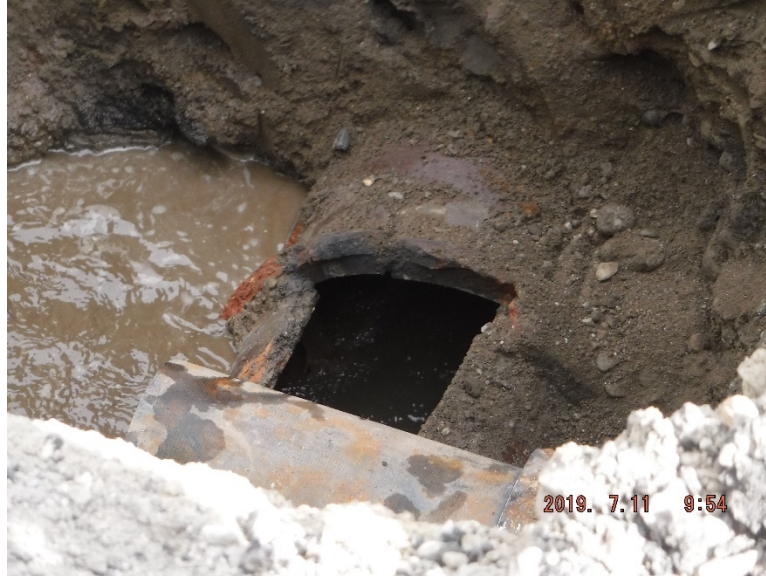
Figure 16: Condition of Haggin storm main, discovered during water main replacement July 2019.
