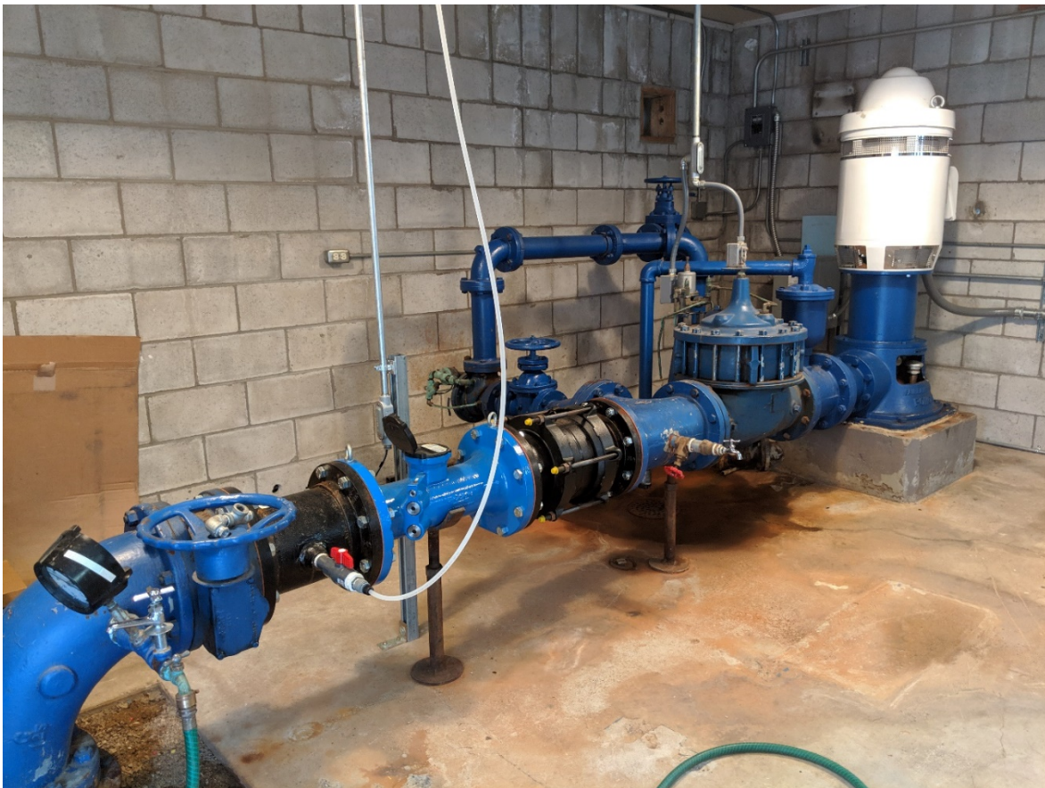
Figure 3.2: Grant Well (Well No. 1)
