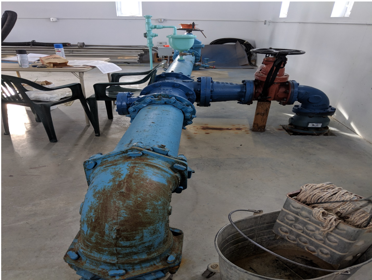
Figure 3.3: Water Plant Well Header (Wells 2 and 3)
