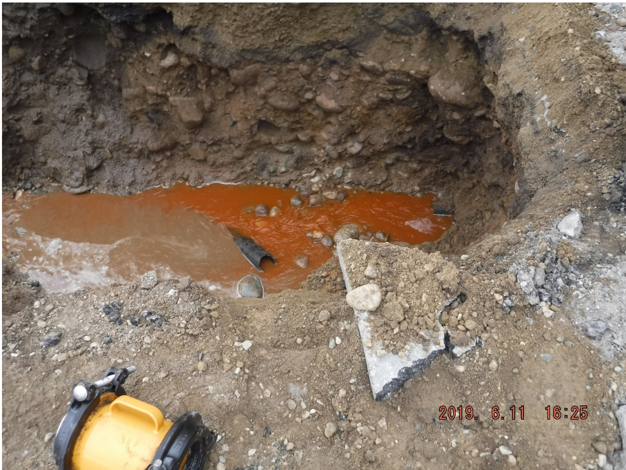
Figure 3.9: Cast Iron Water Main
