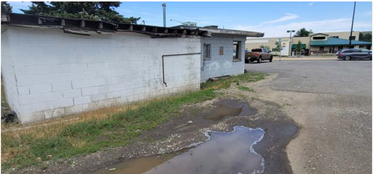
below- an abandoned building with inadequate storm drainage at the southwest corner of Highway 212 and 2 nd street
