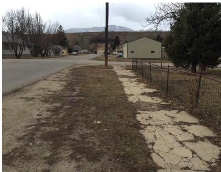
EXAMPLE OF A SIDEWALK IN RED LODGE THAT HAS EXCEEDED ITS USEFUL LIFESPAN (APPROXIMATELY 50 YEARS) AND SHOULD BE REPLACED.
