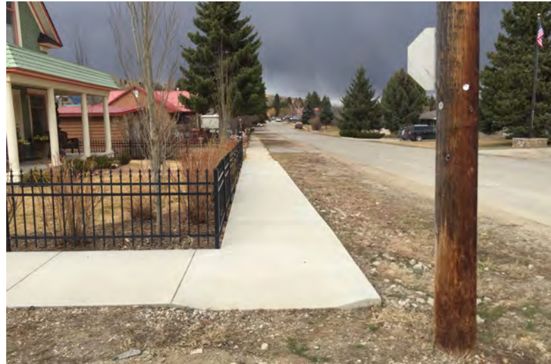
EXAMPLE OF A RELATIVELY NEW SIDEWALK INSTALLATION THAT DOES NOT ACCOMMODATE A SAFE, STREET INTERSECTION CROSSING FOR THOSE WITH LIMITED MOBILITY OR DISABILITIES.
