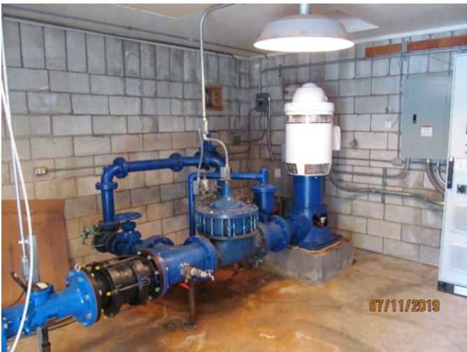
Reconditioned and rebuilt-VFD
