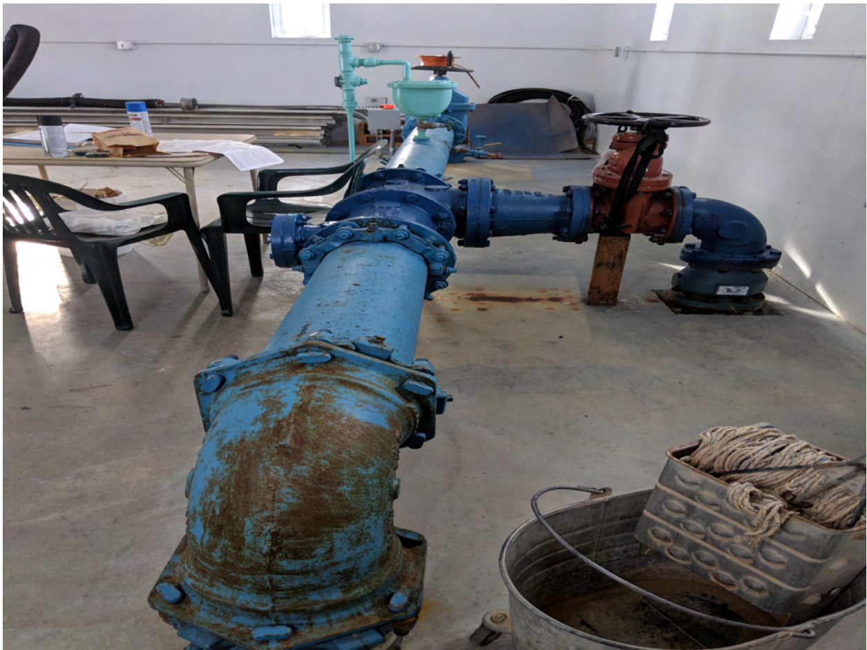
Figure 3.3: Water Plant Well Header (Wells 2 and 3)
