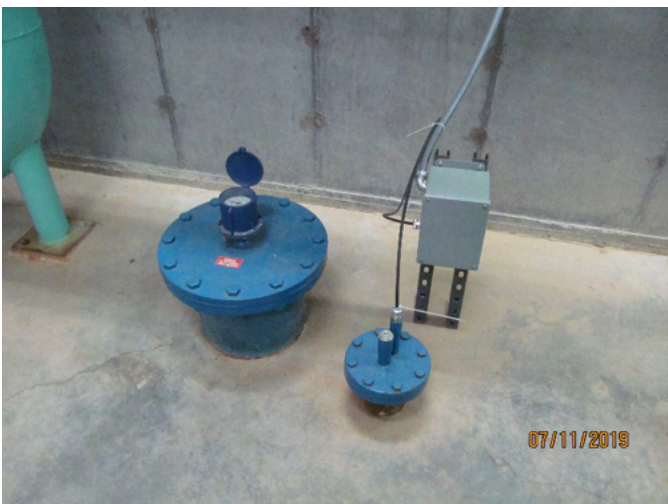
A transducer calls for the well(s) by clearwell level
