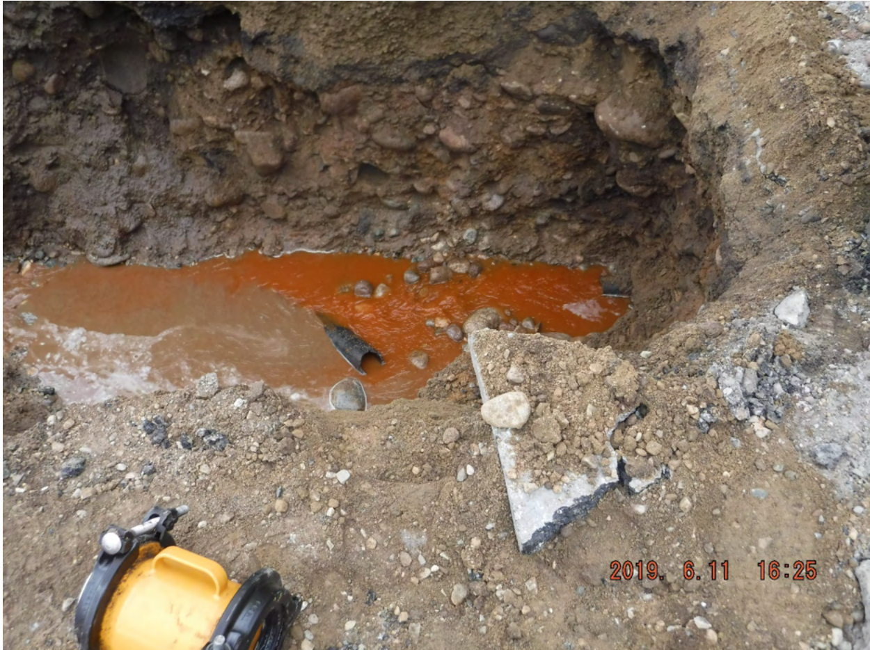
Figure 3.9: Cast Iron Water Main
