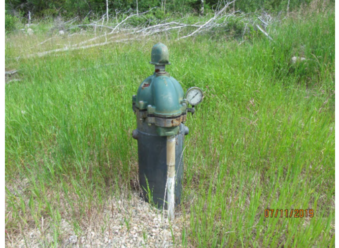
(WL004) Well 3 RLPWSW2 GWIC 223132 -This well is not being used
