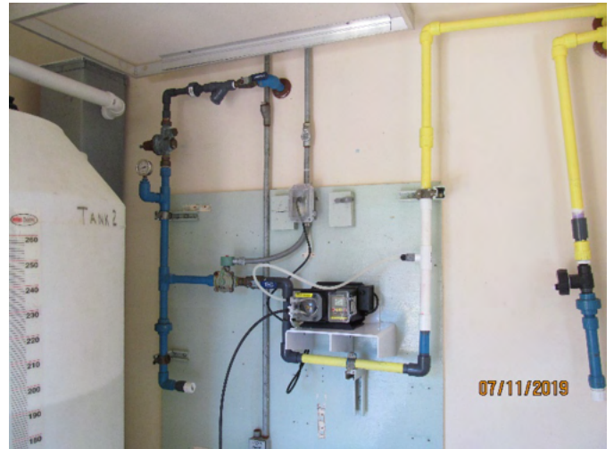
(TP003) Treatment plant well 2, 3
