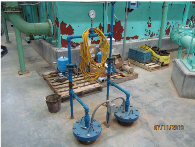
Submersibles provide carriage water for chlorination from the clearwell
