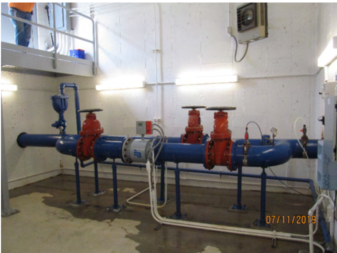
Water leaving is metered and a...
