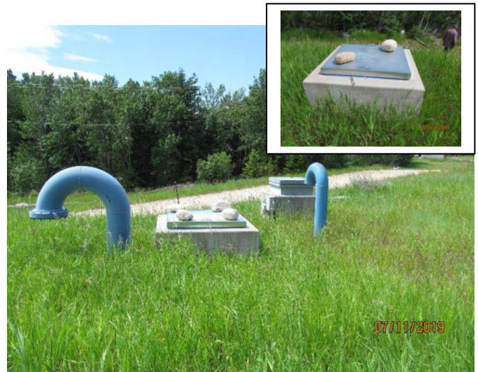
(ST003) Storage tank 3-500,00 gallons-two hatches (bilco), screened vent
