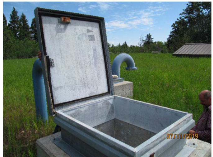
(ST002) Storage tank 2-250,000-single hatch and screened vent
