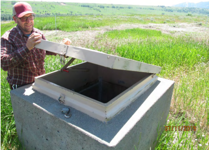
Hatch weather stripping needs attention
