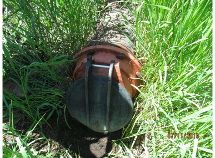
Overflow has a flap gate
