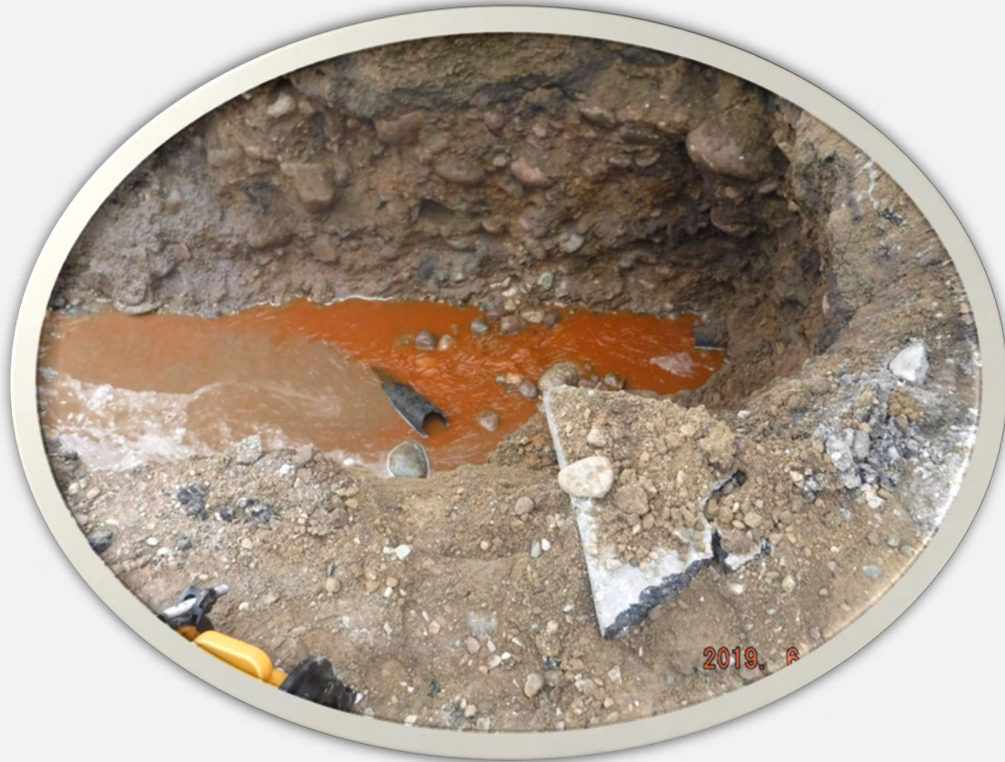
Haggin Avenue Cast Iron Main
