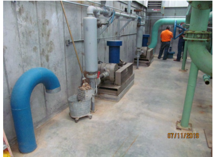
Water then leaves the clearwell headed for storage tanks
