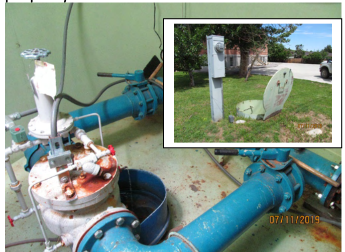
Water on 12 Inch main to town and tank is controlled via this 6 Inch PRV that tank level of Airport (ST001) 750,000 gallon controls
