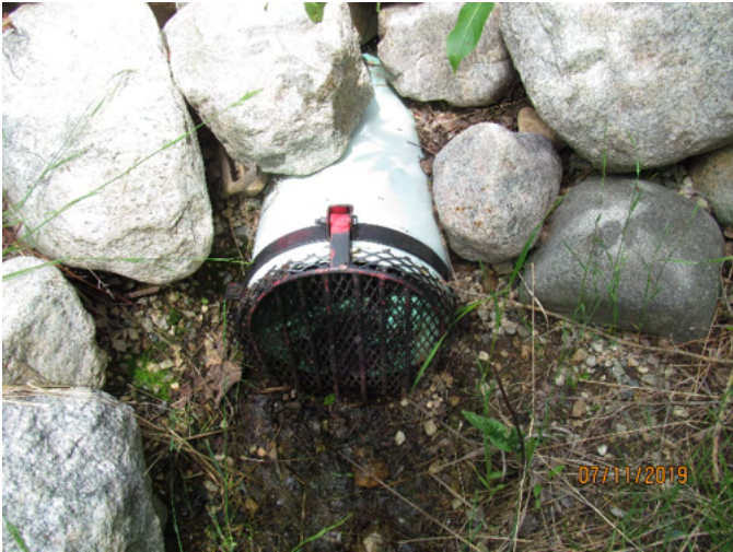
Tanks share common overflow-fixed with flap gate screen
