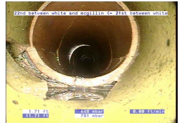
▲ Hole in bottom of pipe where sewer exfiltrating
