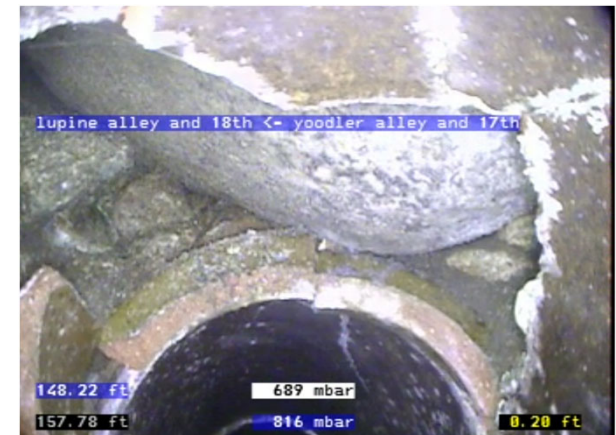
▲ Huge Hole and Boulder in Sewer Pipe
