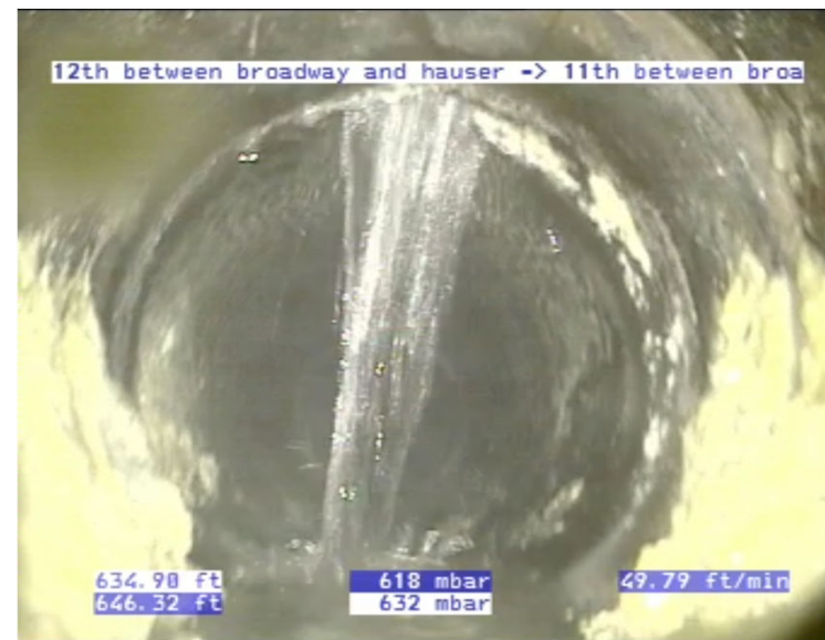
▲ Infiltration Gushing Through Pipe Joint
