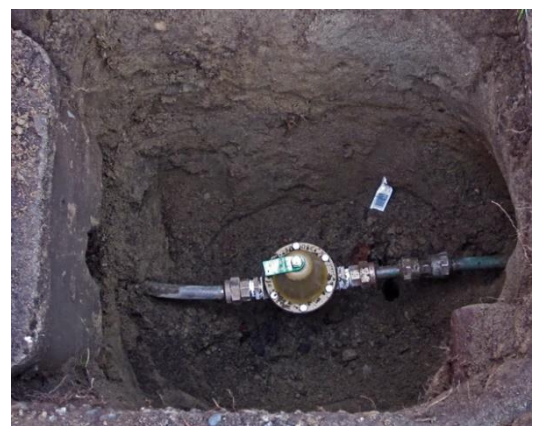
An example of an installed PRV
