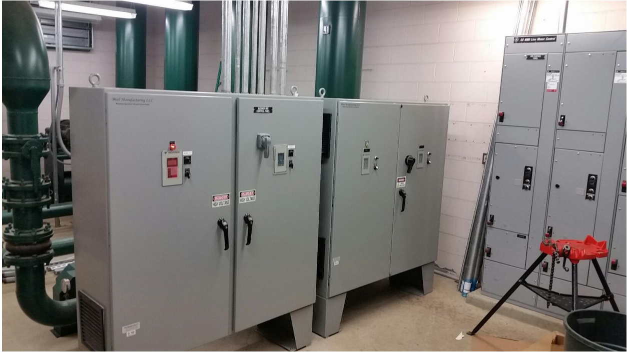
Two of the new Variable Frequency Drives at the Wastewater Treatment Plant
