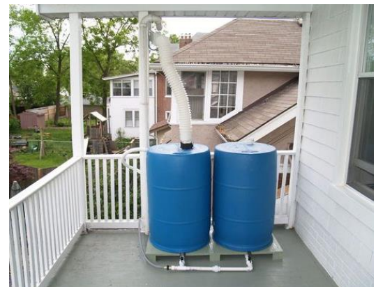
Rainwater collection system at a residential home
