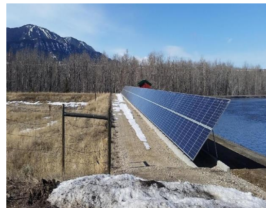
Solar array at the Wastewater Treatment Plant
